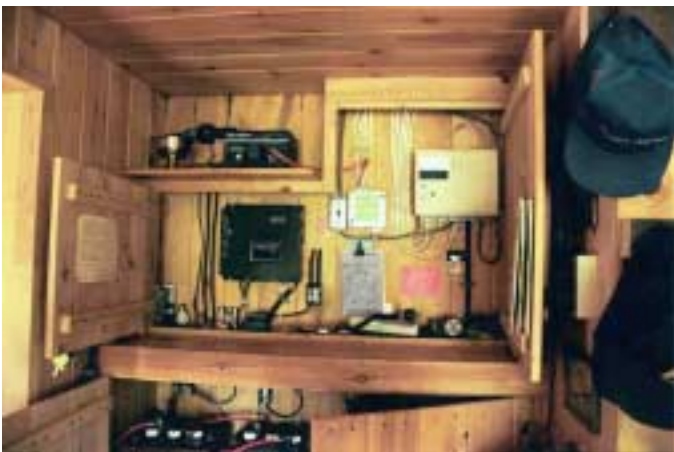
Photo 2 – Hoffman energy center with solar panel controls, batteries and inverter.
