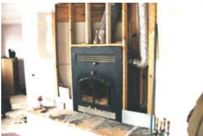
Photo 3 - Jewett zero-clearance fireplace in unfinished living room of house.
